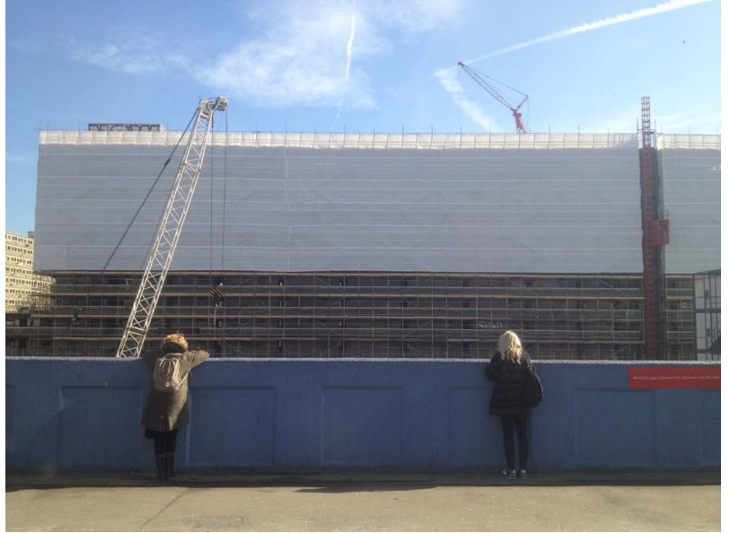
Fig. 7. Heygate banner installed, 15 October 2013. Courtesy of Gary Kinsm Claydon block just after start of demolition, 5 March 2014. Author's own photograph.
