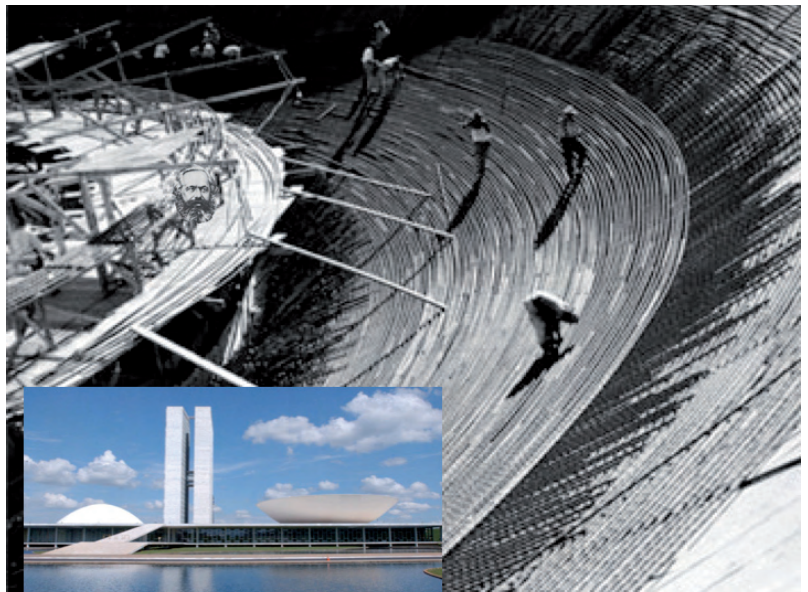
Fig. 6. A typical informal building site with no hierarchy at Agglomerado da Serra, Belo Horizonte, Brazil. Photos and Collage: MOM, 2007.
